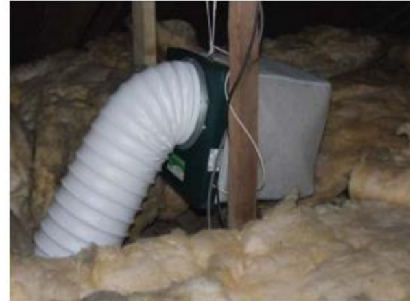
Figure 1: Roof-located positive ventilation system
